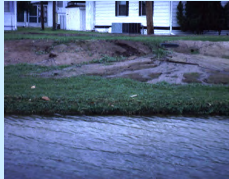
Failing septic tank
