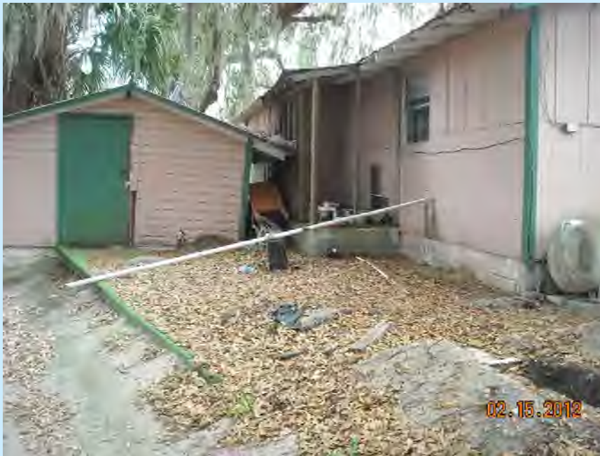
Washing machine discharge
