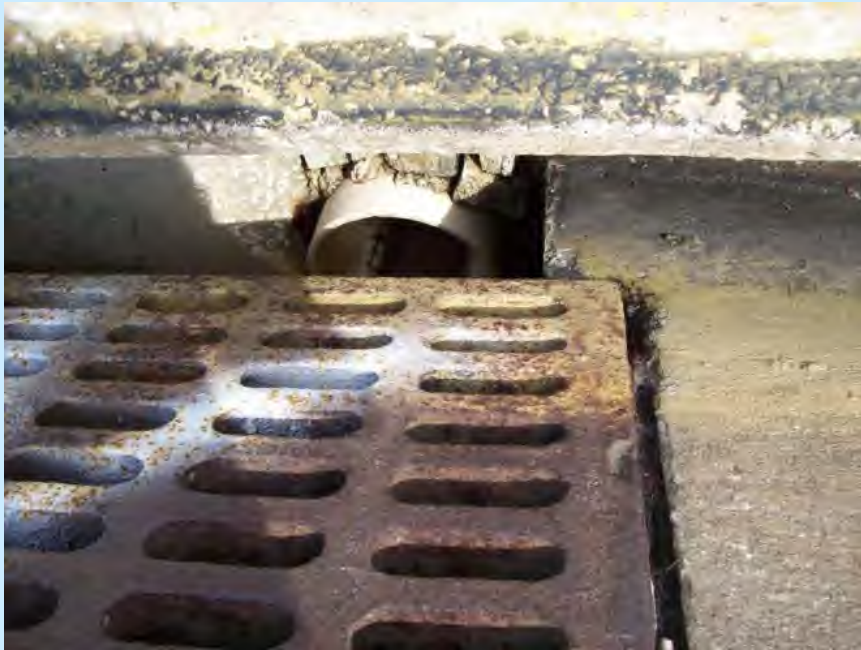
Unknown pipe into storm sewer inlet
