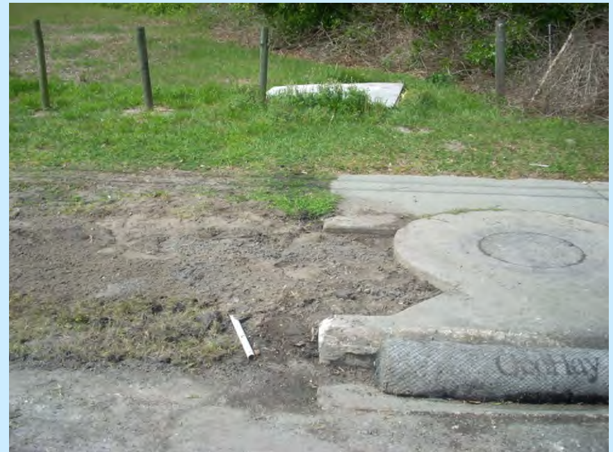
Unknown pipe to inlet
