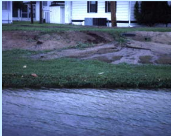
Failing septic tank
