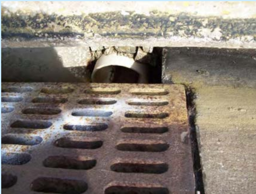
Unknown pipe into storm sewer inlet
