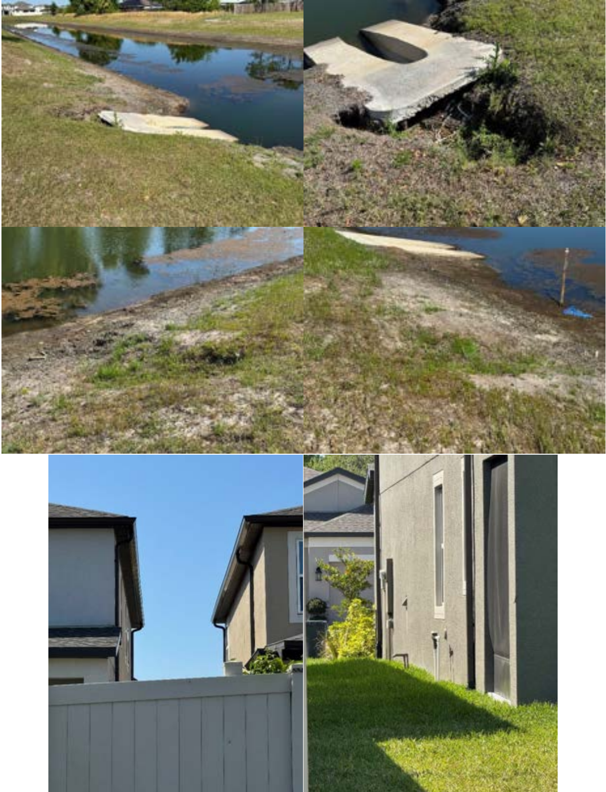
Photo 3 - Displays images of the erosion occurring at Pond E, erosion around the MES drain inlet and gutter system examples.
