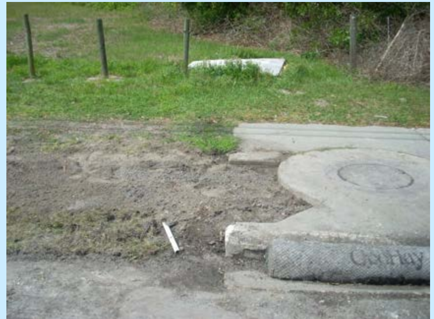
Unknown pipe to inlet
